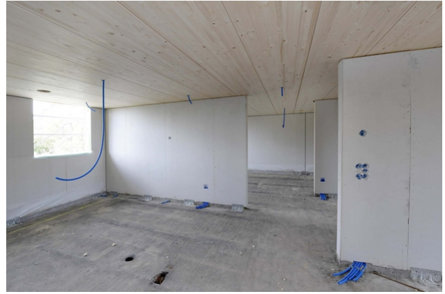
Interior view at the construction site with the floor ceiling in wood
