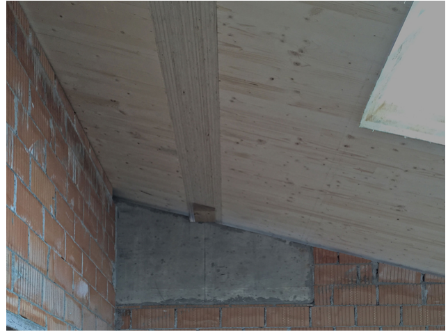
Invisible from below: The Kerto center purlin was integrated into the roof structure
