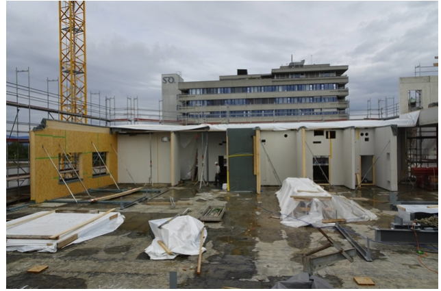
Erected interior wall elements with the prepared recesses for the many installations
