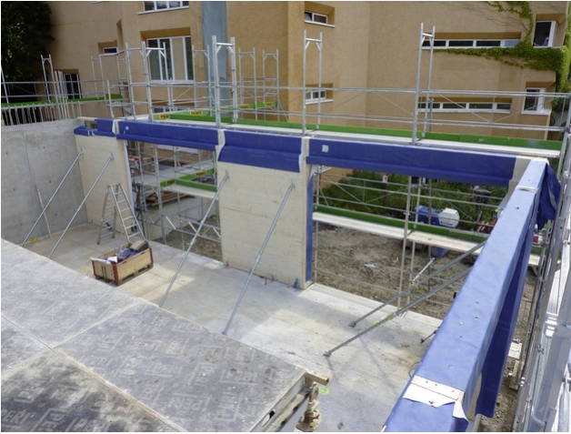
Under construction: first the wooden elements were installed, then the ceilings were concreted
